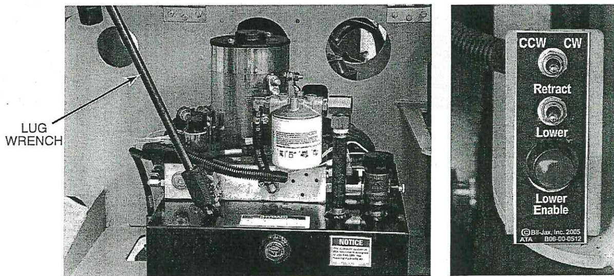
Figure 3-10. Hand Pump and Switch Panel for Auxiliary Operations
