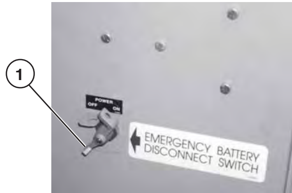
Figure 2-2. Emergency Battery Disconnect Switch
