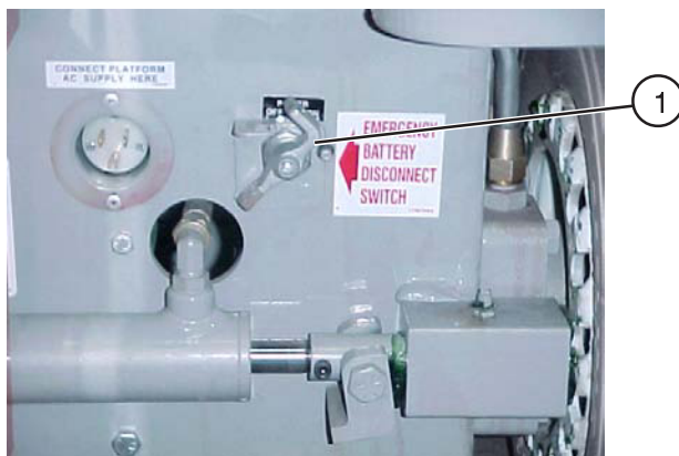
Figure 2-2. Emergency Battery Disconnect Switch
